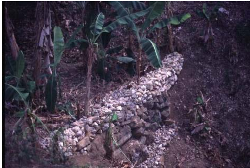
This gully plug, built with rocks, was built by a farmer to capture eroded soil and use the flow of rainwater.
