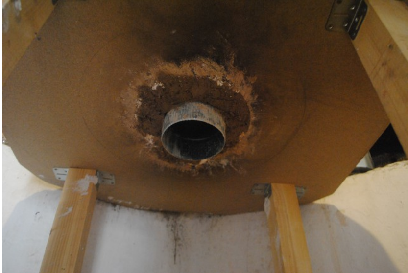
Figure 8. 15cm diameter pipe and 20cm long connecting the stove with the oven. Gaps sealed with mud with some plaster.
